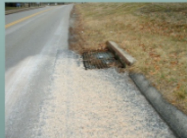
Salt near storm drain
